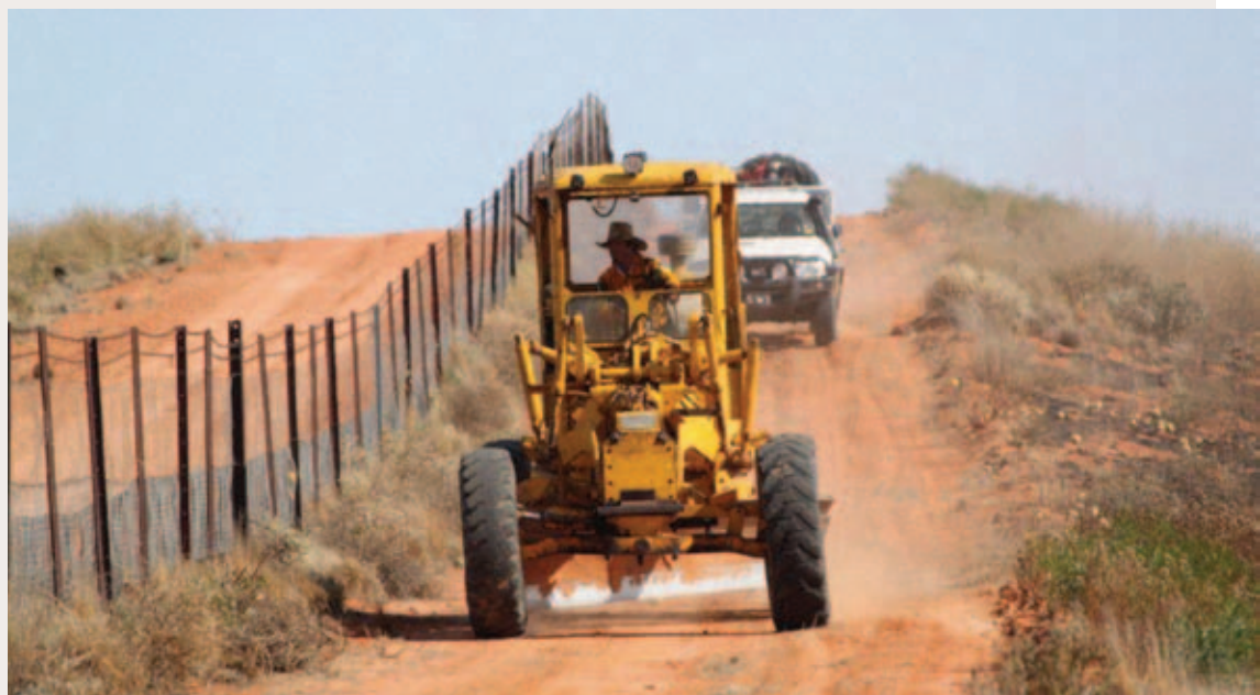
ABOVE: A grader working along the dog fence, building containment lines on the NSW/SA border. Photo by Mark Lacy.
